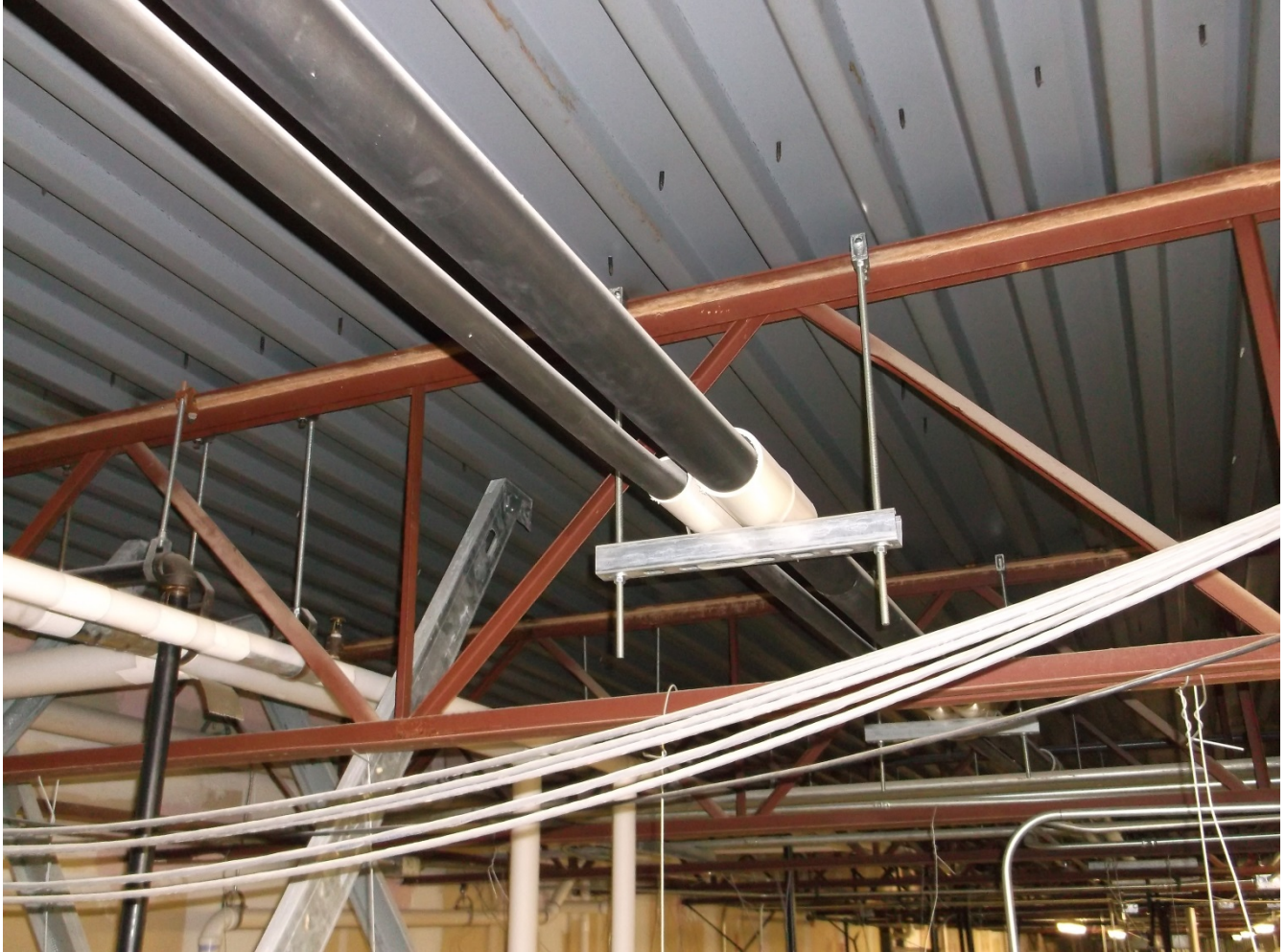
Photo #4 – Exposed rear corridor ceiling. The ceiling was covered with mechanical and electrical piping, along with other hanging fixtures.
