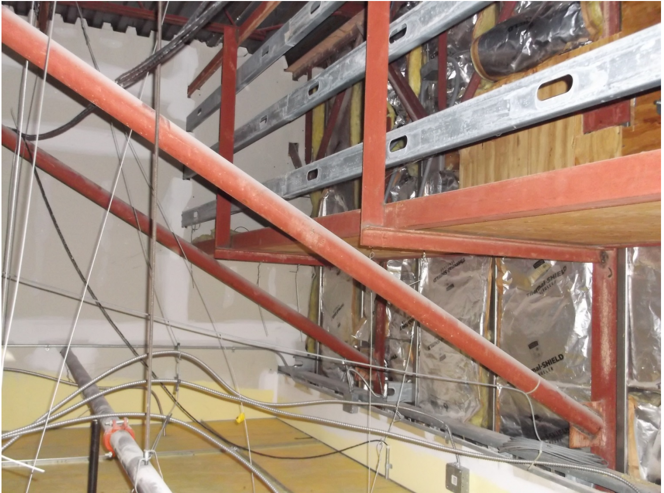
Photo #6 – Inside front storefront wall was an access platform servicing the front of the building. Steel vertical beams with 3” diameter pipes extended back at each joist location – around 5’-3” on center.
