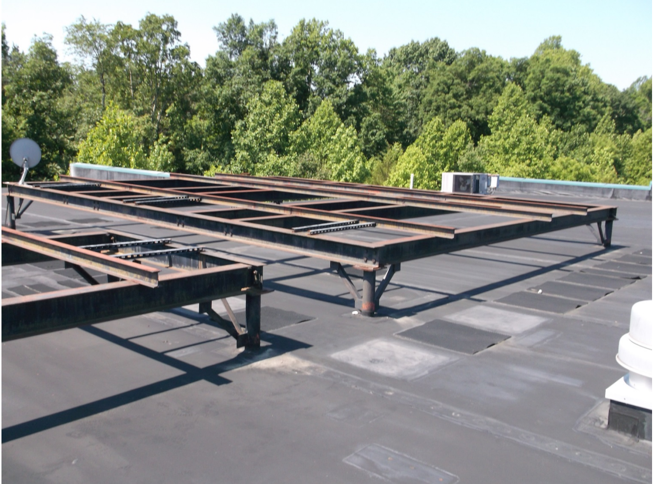
Photo #10 – Steel Beams and Angles that held old RTU’s in back of the Marketplace.
