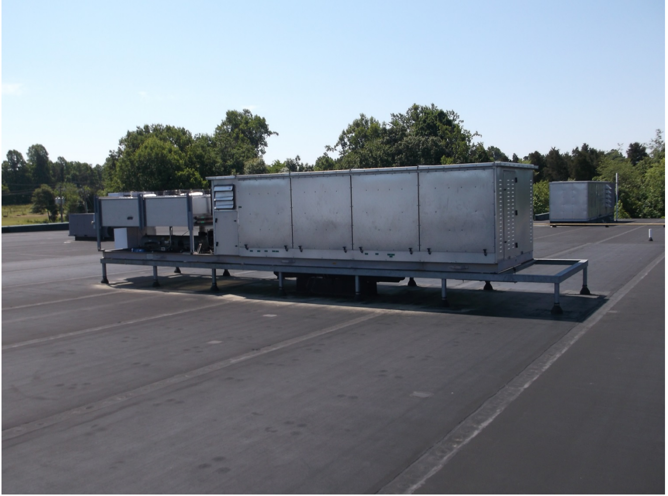
Photo #9 – Kysor/Worren Refrigeration Unit at the front of the proposed Dollar Tree store.
