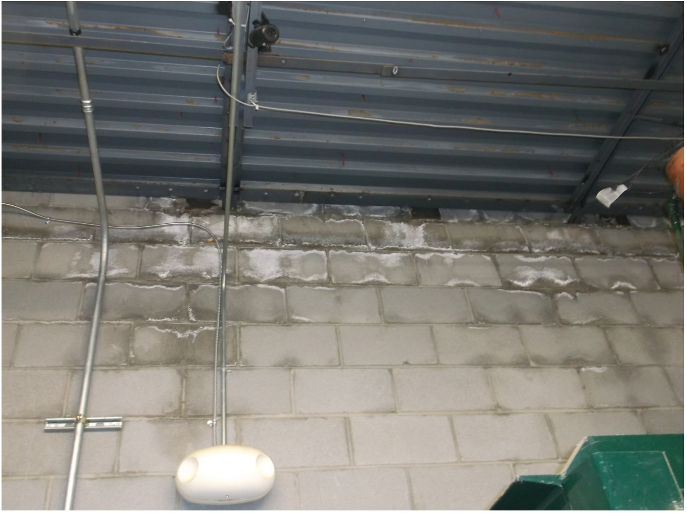
Photo #2 – Effervescence in the back loading dock areas on the concrete walls. The effervescence seems to be concentrated in the wall opposite to the loading dock overhead door. This was an additional that Walmart provided when they took over this space.
