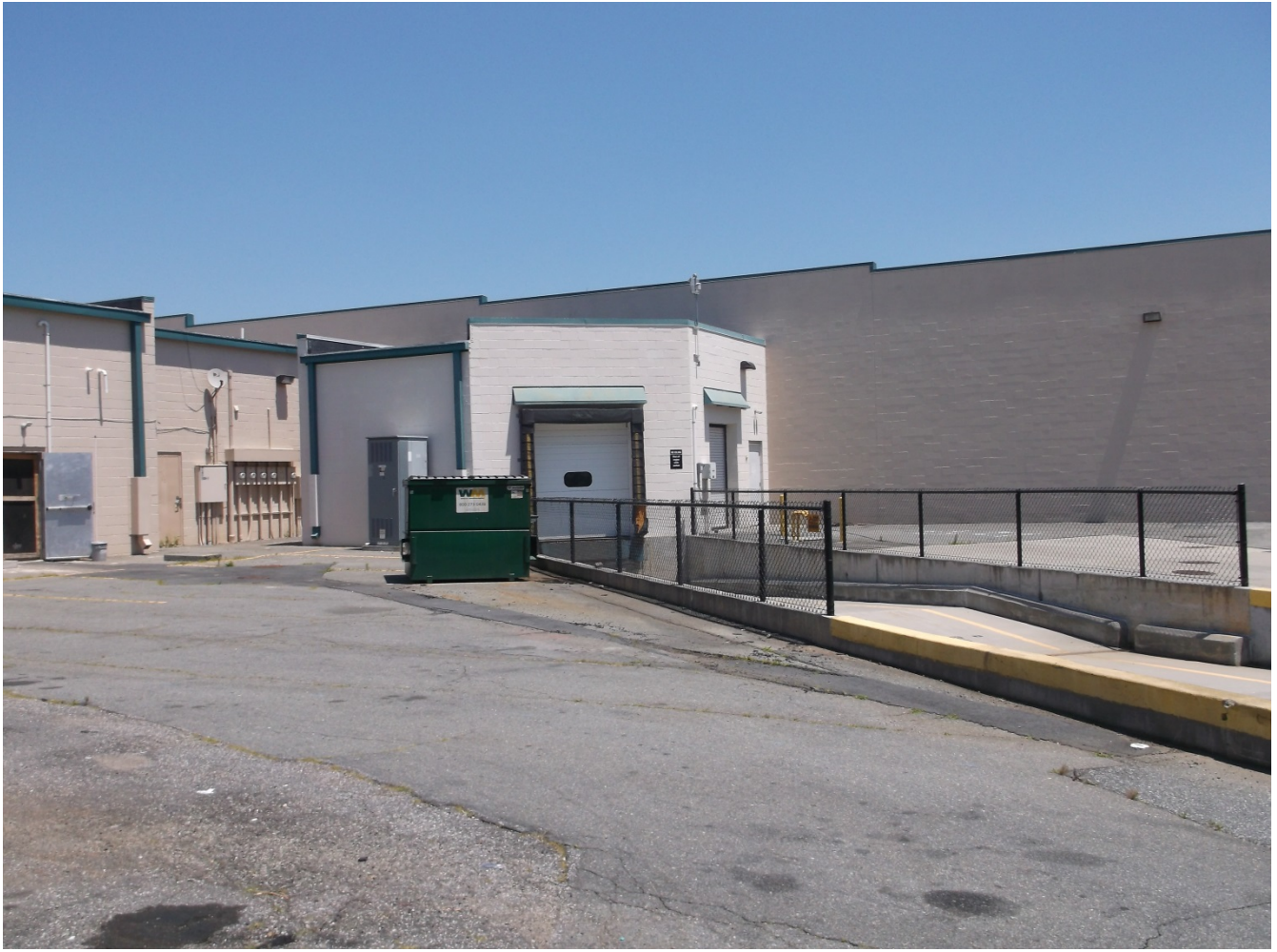
Photo #11 – Loading Dock Ramp located in the back of the Marketplace. There is sufficient room for trucks to maneuver and back into the loading dock. The ramp drops roughly 18” – 24” from the ground surface.
