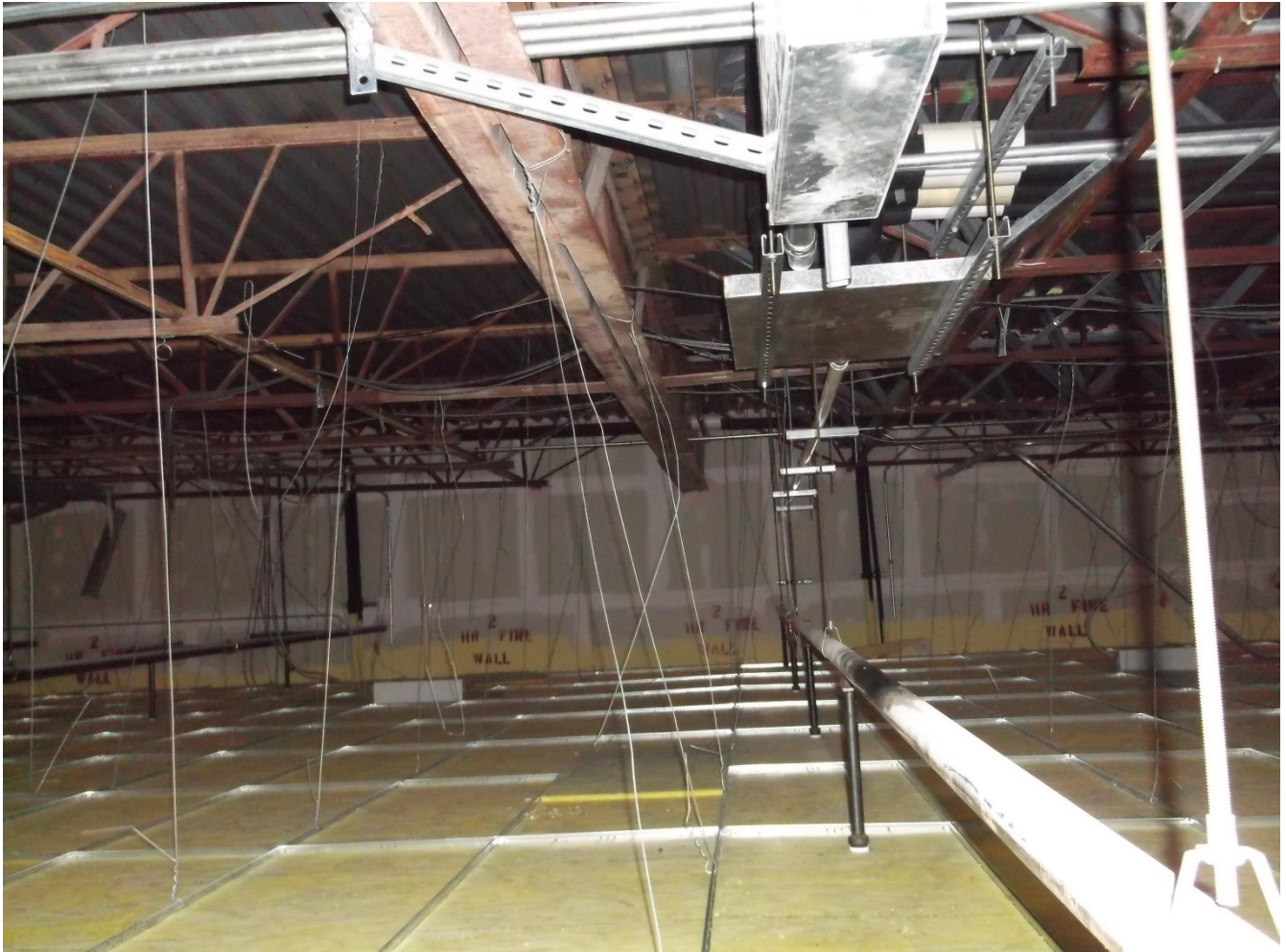
Photo #3 – Steel joist girders extending from side to side of the retail space. Once the joists reach the first column line in the proposed Dollar Tree, the steel joist depth increases from 24” to 44”, due to the RTU’s and other ceiling fixtures on that side of the building.
