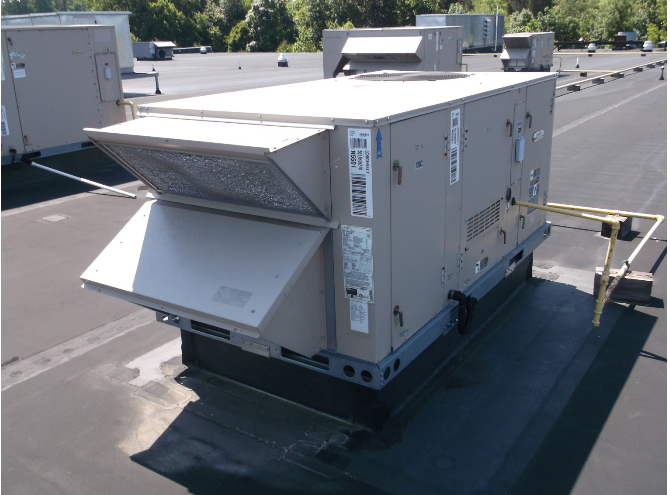
Photo #7 – Existing Lennox RTU’s above the proposed Dollar Tree Store. Two of the newer RTU’s appeared to be in good condition.
